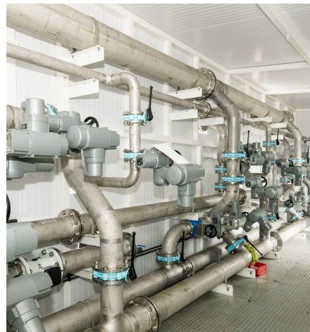
Internal pipework and mechanical installation
