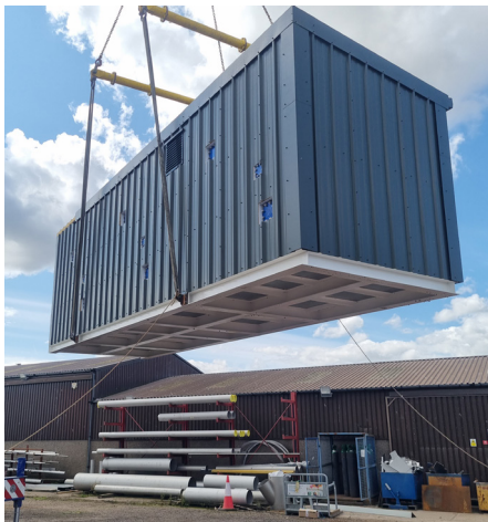
One of the modular units being lifted out ready to be transported to site
