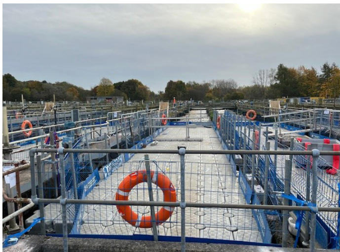
One of the pontoons at the wastewater treatment plant in Bolton
